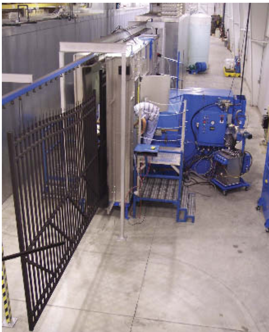
The entire powder coating system runs along a 410-foot-long closed loop. The design incorporates a split zone that can process a 7-foot-tall or a 10-foot-tall part window.
