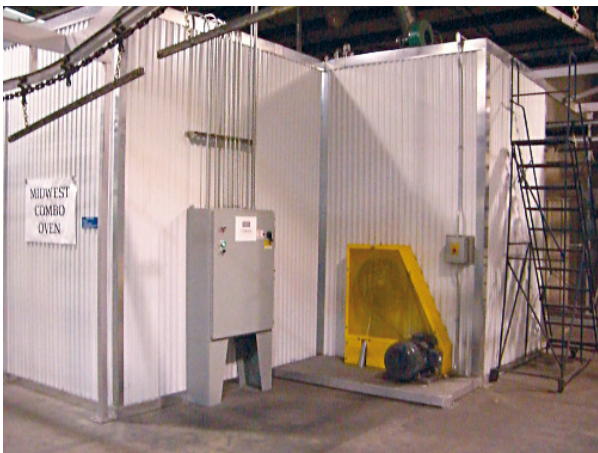
Various close-up views of the powder coating system installed at WireCrafters are seen above.
